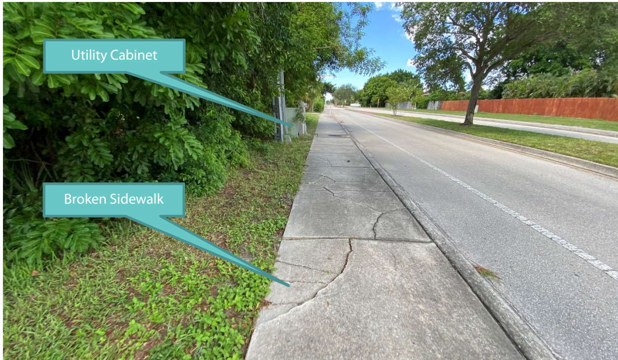
Figure 24: Broken Sidewalk along 75th Street (looking north)
