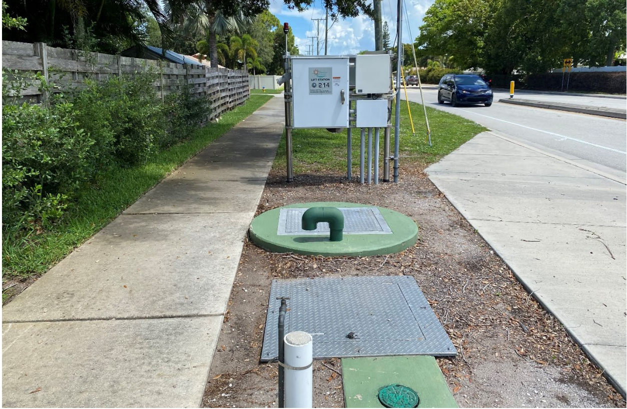
Figure 18: Manatee County Sanitary Lift Station (looking north)
