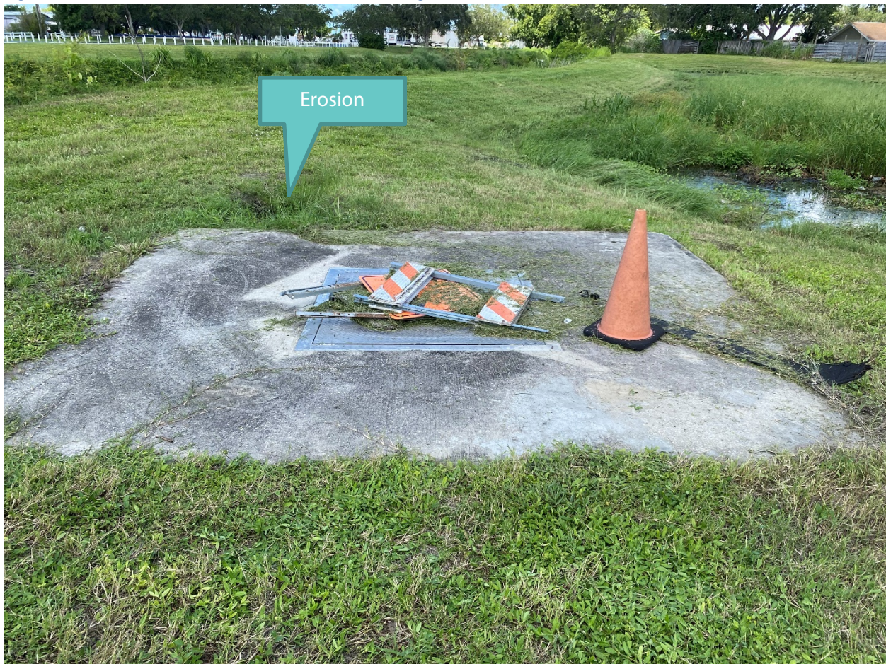
Figure 23: Smartbox Outfall Control Structure (looking west)
