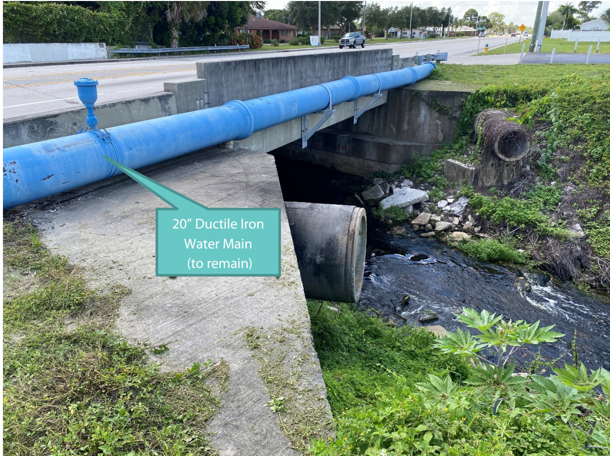
Figure 37: Water Main on Bridge (looking southeast)
